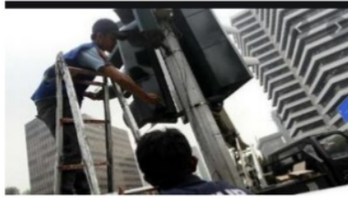
Figure.2 Traffic Lights Broken
