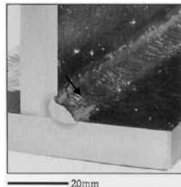
Gambar 12.24 cacat undercut (TWI, 2018)
